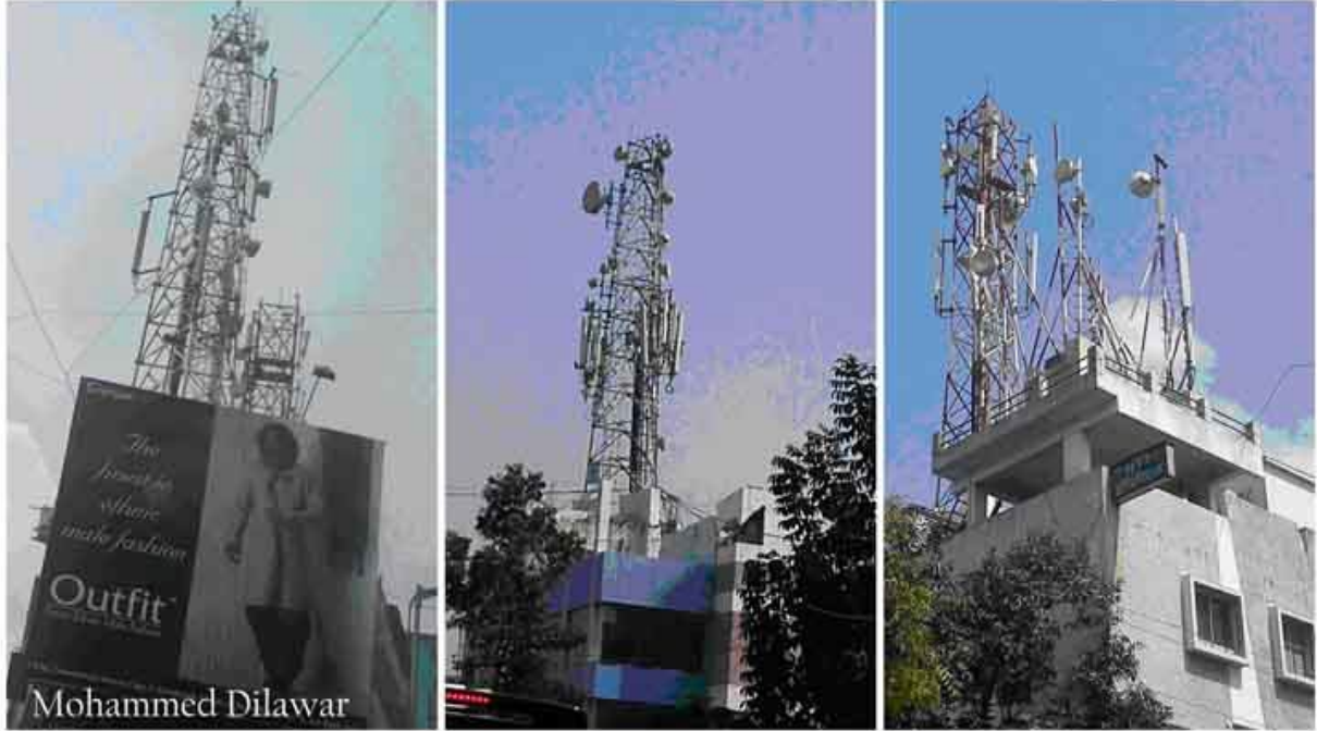
Cell phone Towers on commercial and residential Structures
